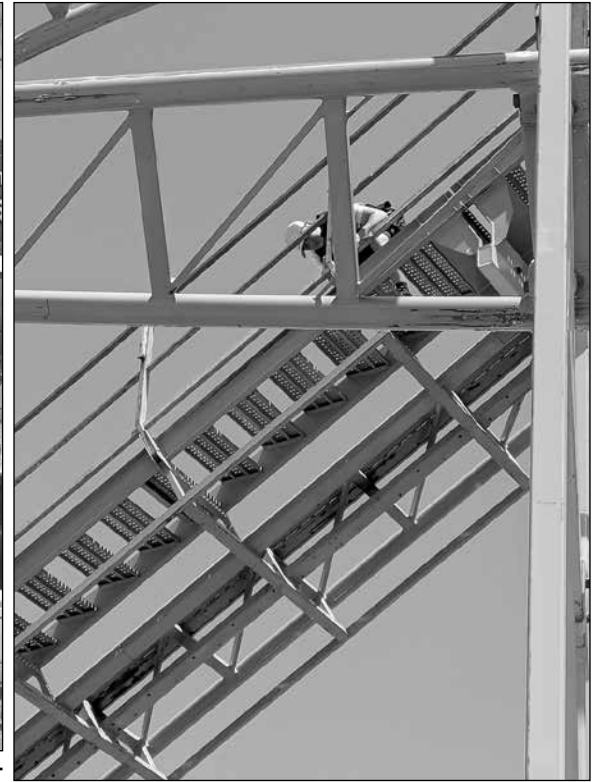
A worker bolts in the last few bolts holding sections of track together on a roller coaster the day before opening day.
