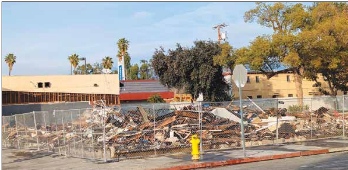
COMMERCIAL BUILDING LEVELED -- An early-morning fire in a vacant commercial structure on Jan. 31 in the 400 block of North Garey Avenue in Pomona destroyed much of the building as seen in the photo above. A Los Angeles County Fire Department spokesperson said the first units were dispatched at 5:24 a.m. and were on the scene at 5:28 a.m. They found heavy smoke coming from the single-story building, upgraded to a second alarm at 5:36 a.m. and knocked down the fire at 7:15 a.m. Nearly 70 firefighters were on the scene. There were no injuries and no indication of a cause. The fire was right across the street to the north of The Union, formerly Pomona's old YMCA.
