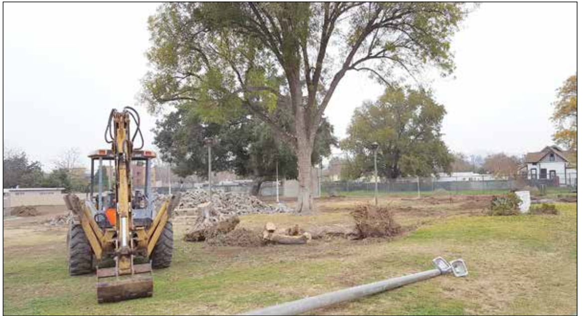
Heavy equipment operators -- working in the rain -- went to work on Monday morning the day after the groundbreaking at Pomona's Hamilton Park. Before the end of the day, the old basketball court, several lighting poles and other fixtures had been cleared for work on the on-going upgrade at the park.
